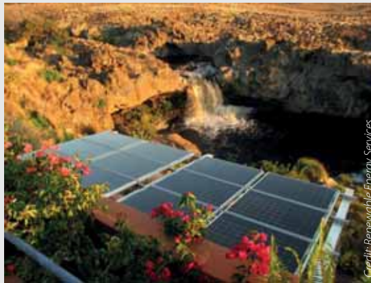
From high-end residential installations today, solar-plus-storage will gradually reach the mass market
