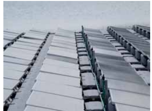
Figure 9. Sunseap/C&T testbed system with active cooling
