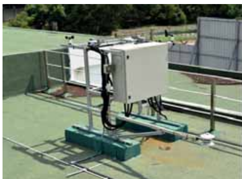
Figure 10. Meteorological station at the rooftop
