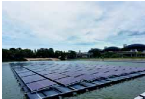
Figure 3. REC/Takiron testbed system
