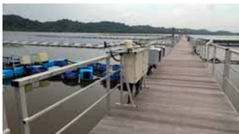
Figure 11. Meteorological station on the floating pontoon
