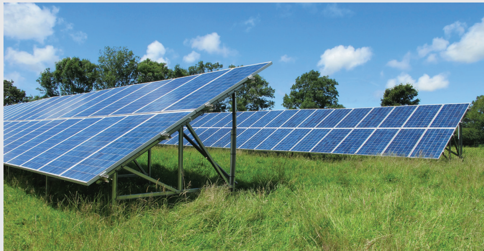
Lightsource has developed a bespoke SCADA system for its growing fleet of PV plants.
